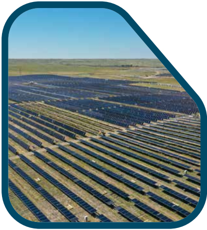
Basin Electric purchases 114 megawatts of output from Wild Springs Solar in Pennington County, South Dakota.
