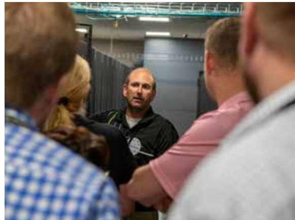
Jeremy Wittenberg, Basin Electric enterprise systems administrator III, leads coworkers on a tour of the data center during an open house event facilitated by the Information Technology team.
