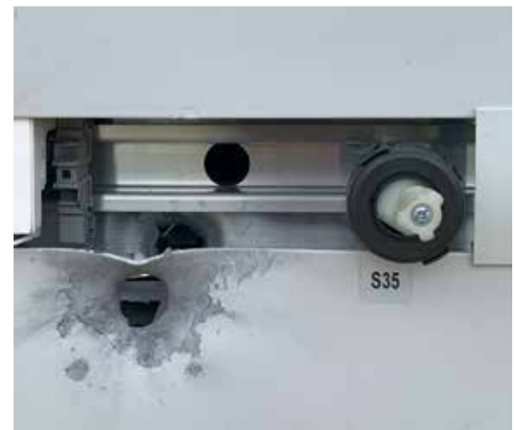
The Wheelock substation sustained damage after Smith fired rounds from a high-powered rifle, resulting in the disruption of electrical services for many.
