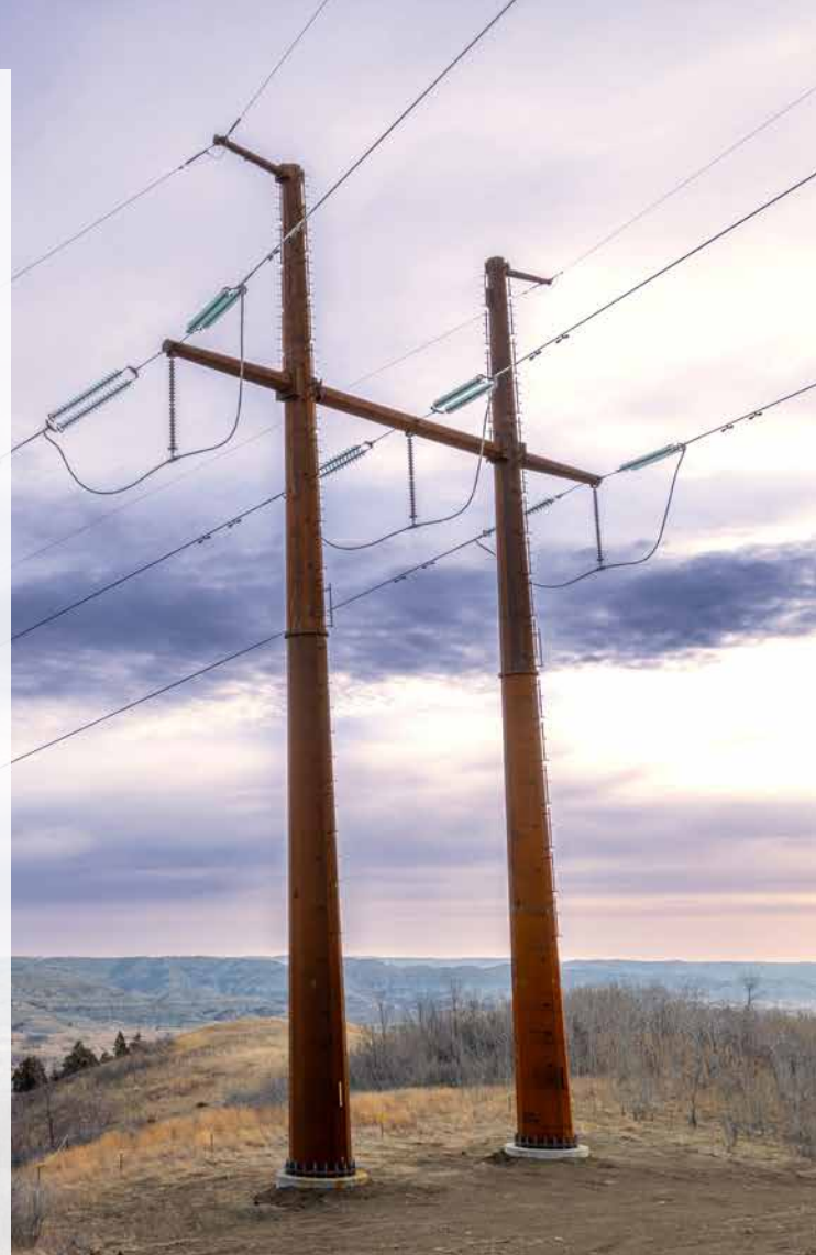
The Roundup-to-Kummer Ridge 345-kV transmission line stands tall against the wide-open skies in northwest North Dakota.
