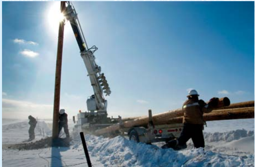
Crews from Cass County Electric Cooperative, Fargo, ND, assist KEM Electric in replacing poles. (Photo by J.C. Balcom of the North Dakota Association of Rural Electric Cooperatives.)
