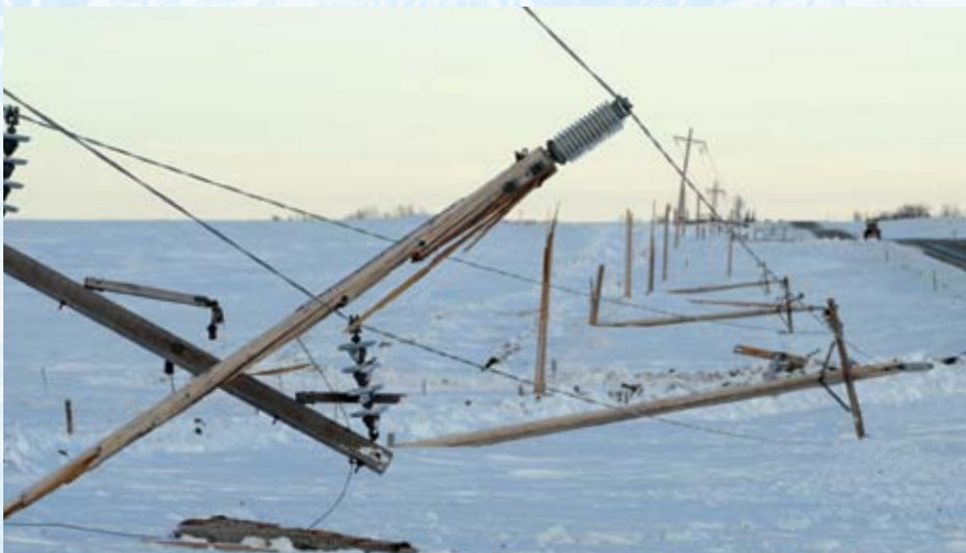
Moreau-Grand Electric Cooperative estimated the weight the ice added to their lines approached 1,200 pounds per 250-foot span. (Photo by Michelle Schweitzer of Moreau-Grand.)
