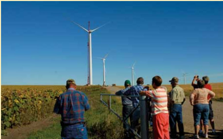
Crews lift one of the last rotors into place at NextEra's Wilton Wind Energy Center on Sept. 23 as members on tour from Crow Wing Power, a Class A member of Basin Electric, look on.
