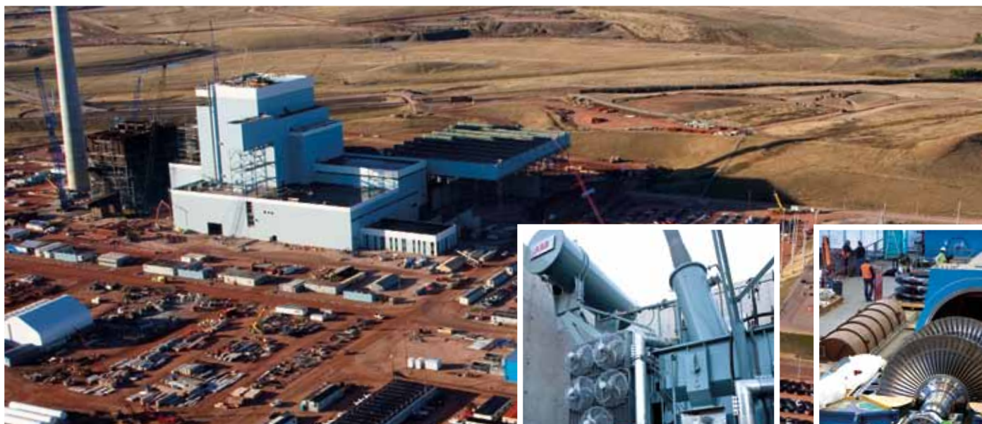
The Dry Fork Station proudly sports its "Basin Blue" siding in this aerial photo taken in September 2009. As of Oct. 1, the project was about 75 percent complete, including engineering, procurement and construction activities.
