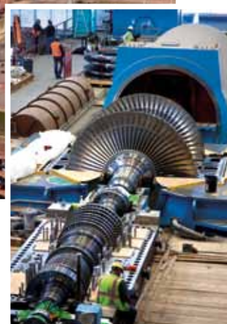
The combined high pressure and intermediate pressure and separate low pressure rotors have been installed at the Dry Fork Station. The power plant is on track for commercial operation in 2011.
