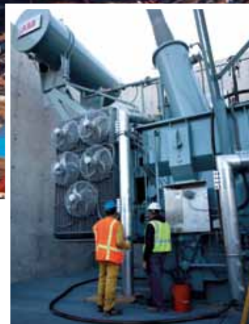
Chairat Phutphong of ABB and Mike Koenig, lead substation electrician from the Wheatland Transmission System Maintenance outpost, prepare to pull vacuum in the reserve auxiliary transformer at the Dry Fork Station.
