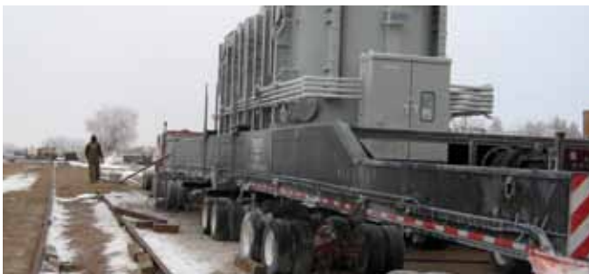
Charlie Creek's new transformer is loaded from the rail onto a truck at Belfield.
