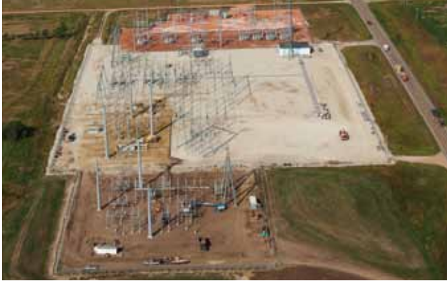
The Charlie Creek Substation near Killdeer is getting a new transformer and a 230-kilovolt bus. The additions support Western's upgrade of their line that heads north out of the substation.
