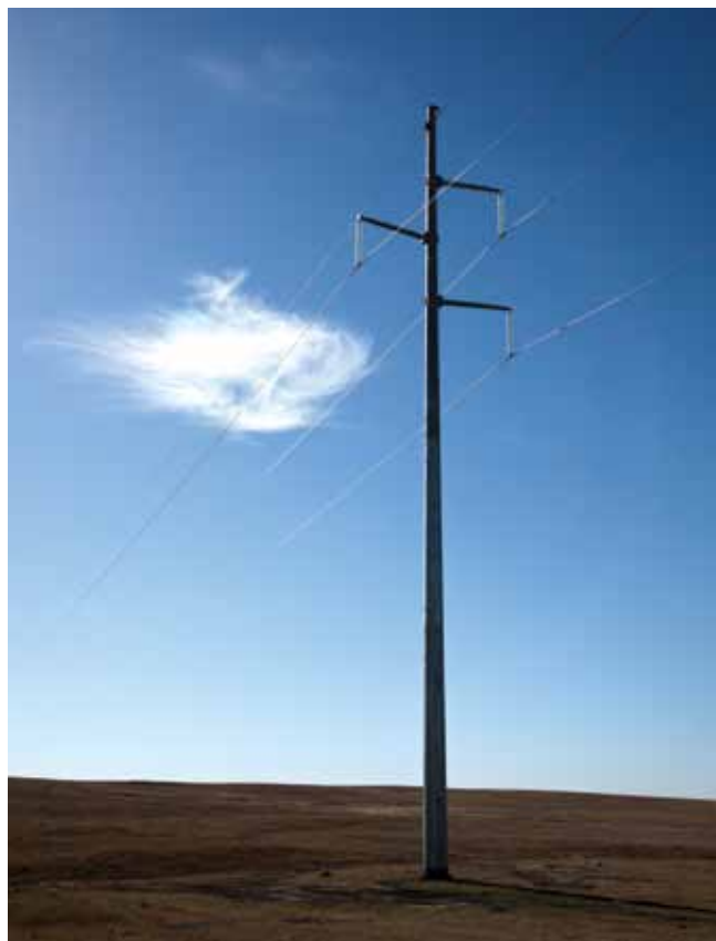
The structures on the new 345-kilovolt (kV) line will be like the ones on the Williston-to-Tioga 230-kV line, shown here, only bigger.
