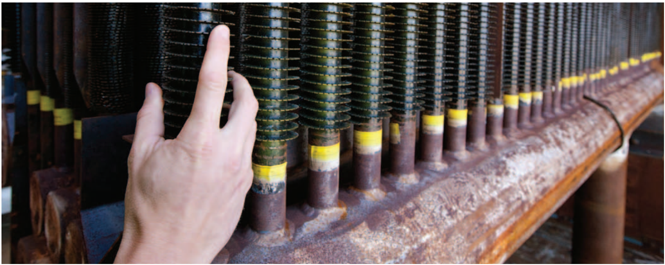
A close up look at the fins on the HRSG module tubes. Each tube is made of different material and each tube's fins are spaced differently, depending on its placement in the casing. The tubes closer to the turbine's exhaust need to withstand more heat than those farther away.
