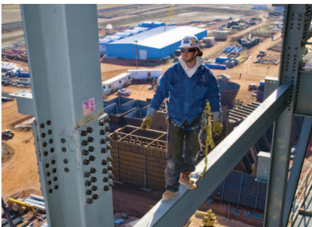
Joe Bowden walks the high steel during construction of Basin Electric's Dry Fork Station near Gillette, WY.
