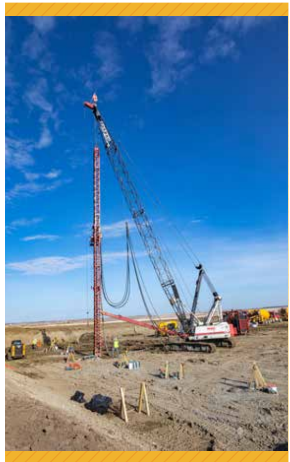
When drilling auger cast piles for ground stabilization, an auger drills down 34-65 feet. As the auger is slowly removed, cement-like grout is pumped down through the center of the auger, backfilling the entire hole. Rebar cages are then installed toward the top of the hole to a set elevation and allowed to cure.
